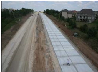
Municipal Paving Award Nall Ave., 143rd St. to 159th St. Leawood & Overland Park, KS
