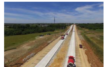
Municipal Paving 159th St. Nail Ave. to Mission Rd. Overland Park, KS
