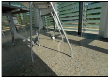
Polished Concrete Galileo's Pavilion, JCCC Overland Park, KS
